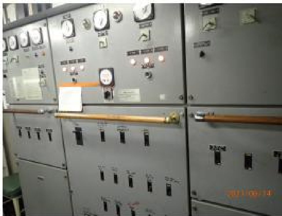
MAIN ELECTRICAL PANEL
